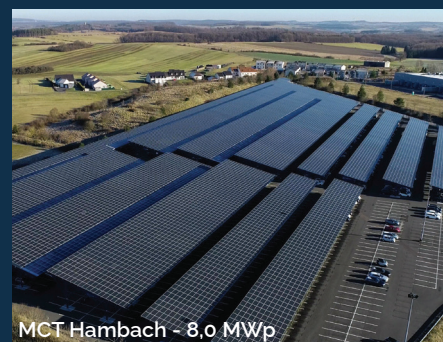
MCT Hambach - 8,0 MWp
